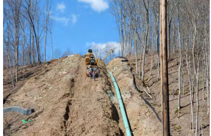
CONSTRUCTION OF OHIO VALLEY CONNECTOR: A 30 INCH NATURAL GAS PIPELINE IN WETZEL COUNTY
